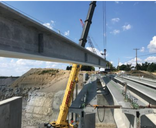
The 72-in.-deep beams were produced with semi-lightweight concrete (125 lb/ft 3 ) to reduce the shipping weight. The beams were placed using one crane on the quarry floor and one crane above on State Route 235.
