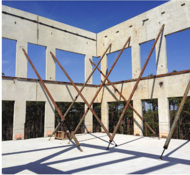
Bracing of a two-story wall panel on the Reserve at Sierra Pines Phase II building is underway.
