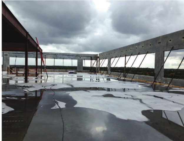
This is a photo of the fifth-floor braced panels at the Offices at Greenhouse, a five-story stacked tilt wall building in Houston.
