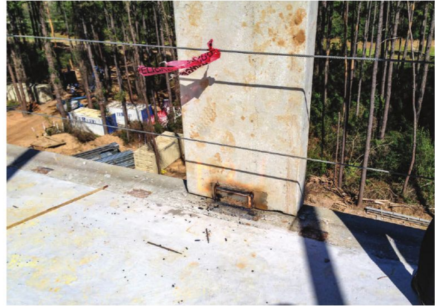
Fifth- and sixth-story panels in place at Reserve at Sierra Pines Phase II building in Houston.
