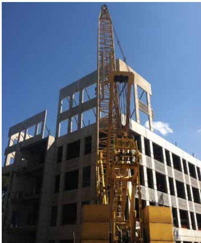
Erection of the upper panels on the northwest corner. Courtesy of Big 4 Steel Services, L.P.
