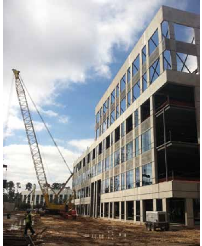
Erection of the upper panels on the east face as viewed from the northeast corner. Courtesy of Big 4 Steel Services, L.P.
