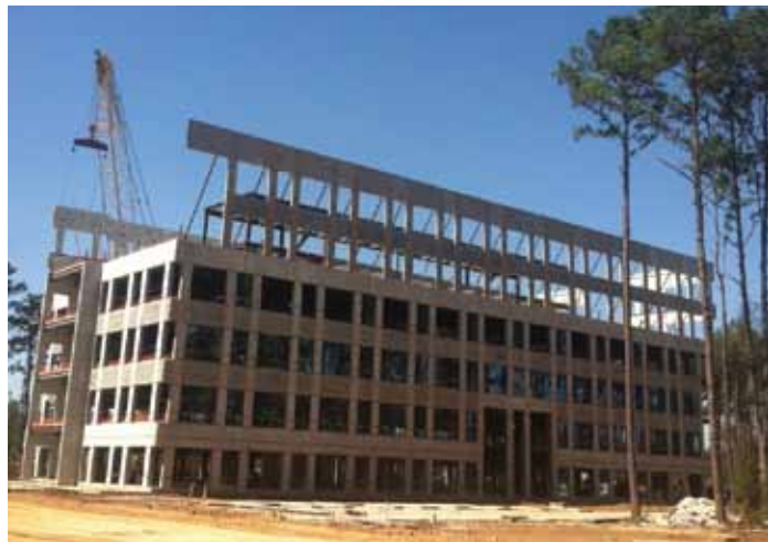
Overall building perspective looking at the east face as viewed from the parking garage. Courtesy of Big 4 Steel Services, L.P.
